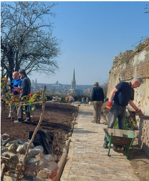
Work in progress on the upper viewing area, new pathway and the sensory garden.
